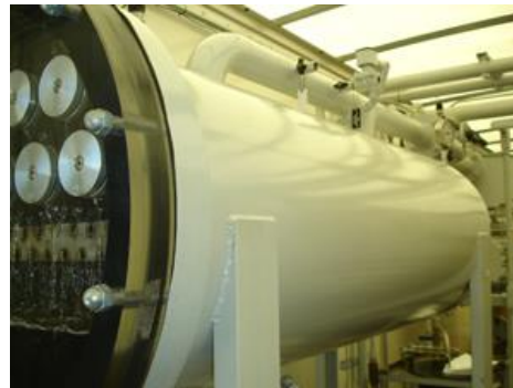
Oil Processing Unit
